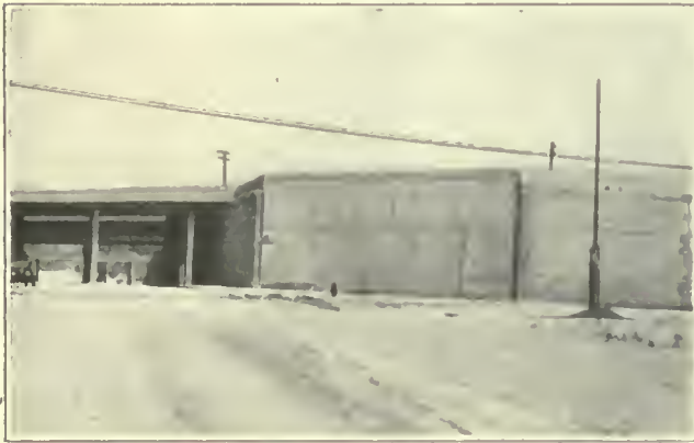
FIG. 276. TRACK ELEVATION. Concrete retaining walls on the Pittsburgh, Fort Wayne & Chicago Railway at 75th Street and Greenwood Avenue.
